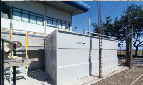
STP at Sports Complex, Brgy. Tunasan
