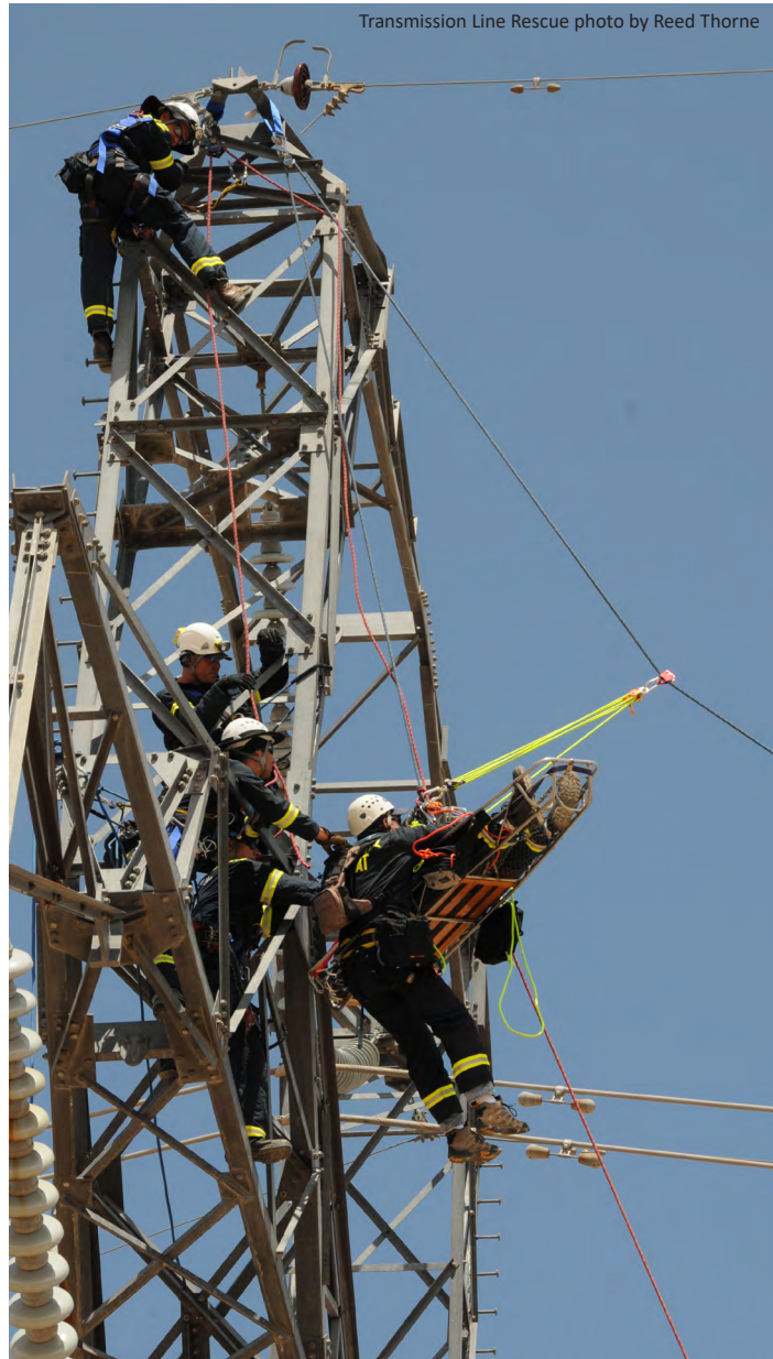
Transmission Line Rescue photo by Reed Thorne
