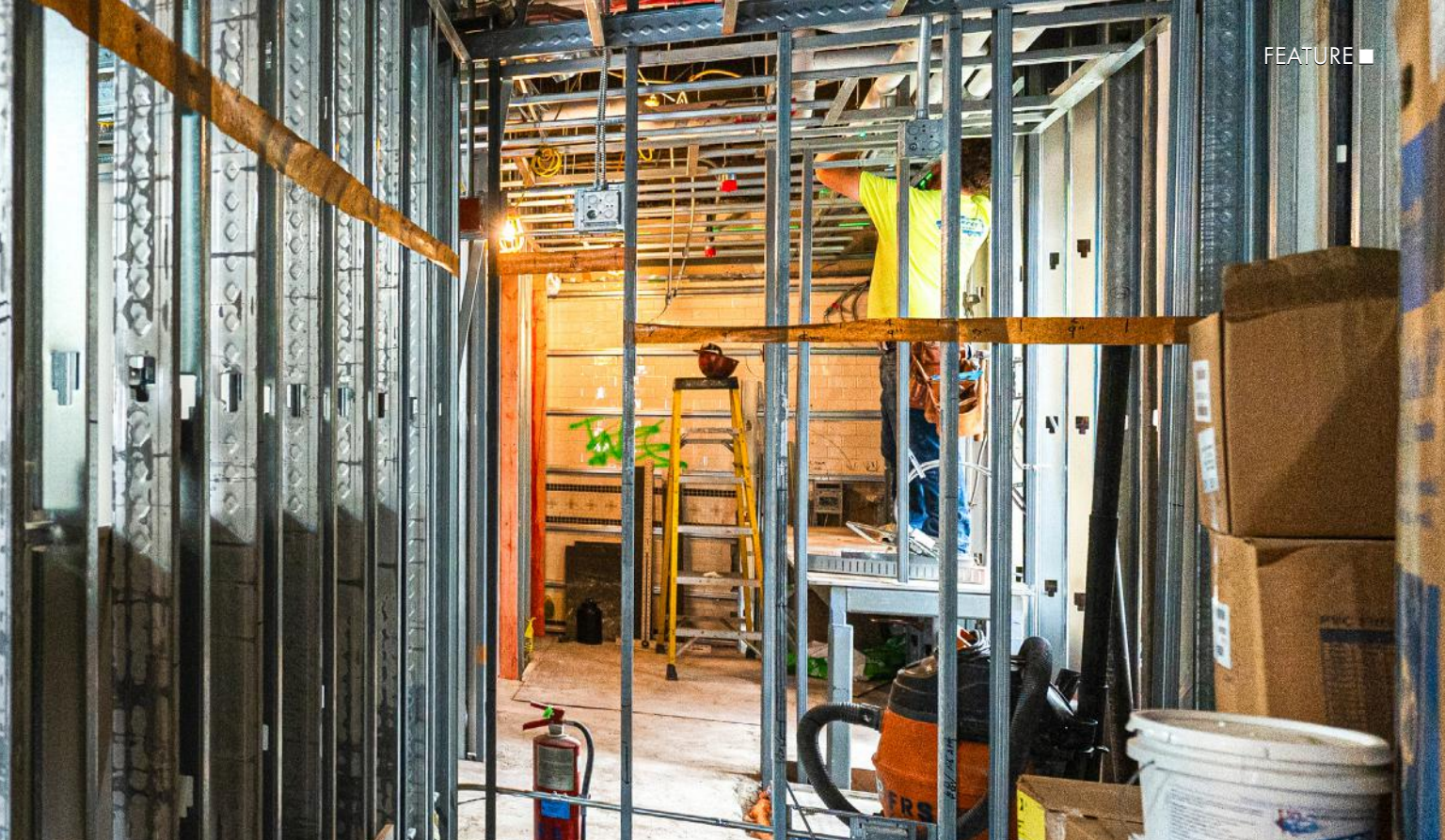
The layout left no room for error—and a tight squeeze for the panels.
