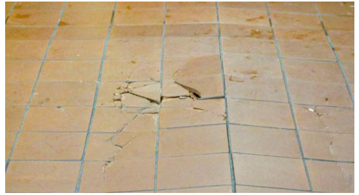
Tile will rebel, as evidenced here, when there is no allowance for expansion and contraction. Properly-designed movement joints will absorb this movement.
