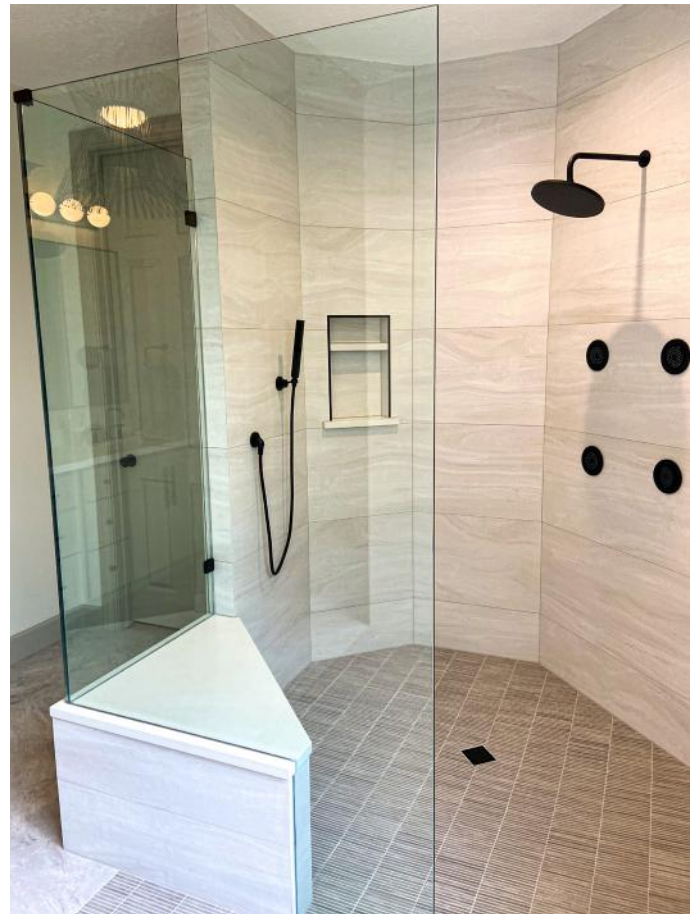
As Owner of Syndicate Tile and Stone, Struzik completed this project with 2’ x 4’ tile on a full LATICRETE system over a mud bed.
