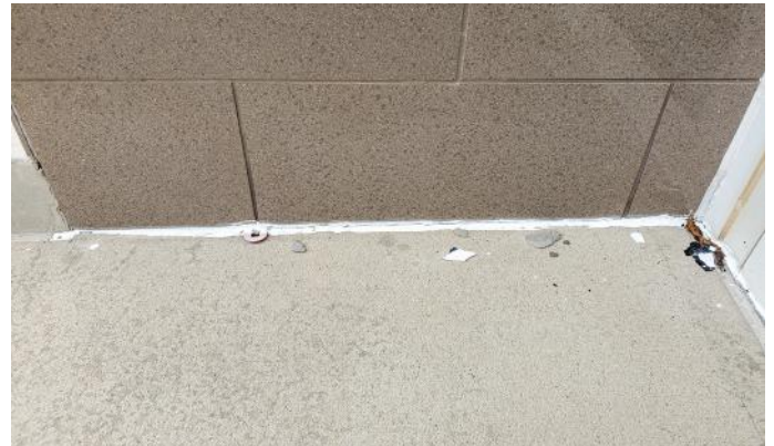
Exterior wall tile also requires movement joints at the change in plane. This image shows a sealant joint (although not well done) between the wall tile and concrete sidewalk.
