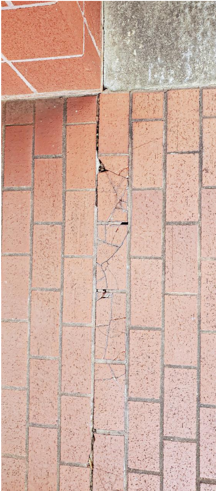
Ongoing maintenance on exterior installations is crucial. When this grouted movement joint fails, water can enter the tile assembly, freeze, and destroy the tile.
