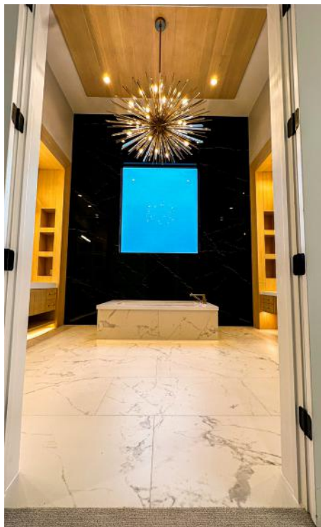
Struzik had to erect full scaffolding to complete this project for Platow Home and Tile, using 6' x3' 3/8"-thick porcelain to a ceiling height of 22' tall.
