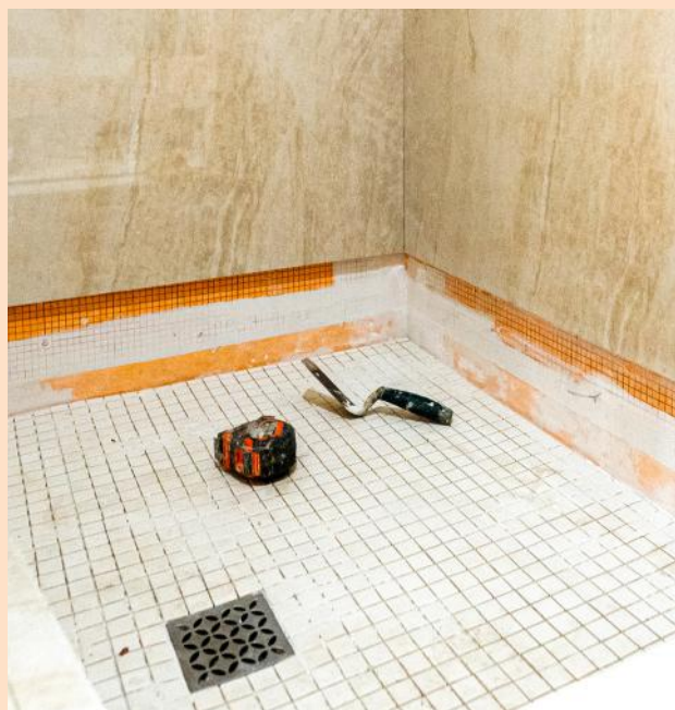
KERDI membrane bonded to mortar bed with KERDI-DRAIN and mosaic floor substrate in place.
