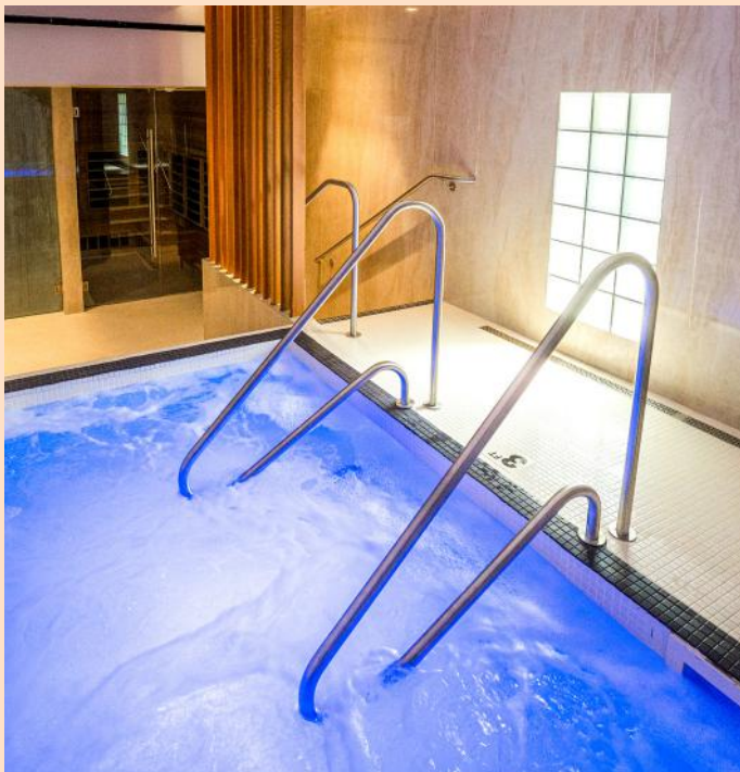
The jetted-tub deck features multiple KERDI-LINE drains installed in tandem for seamless water management.
