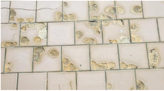
When inappropriate tile is used in freezing temperatures—as seen here—the tile will fail.
