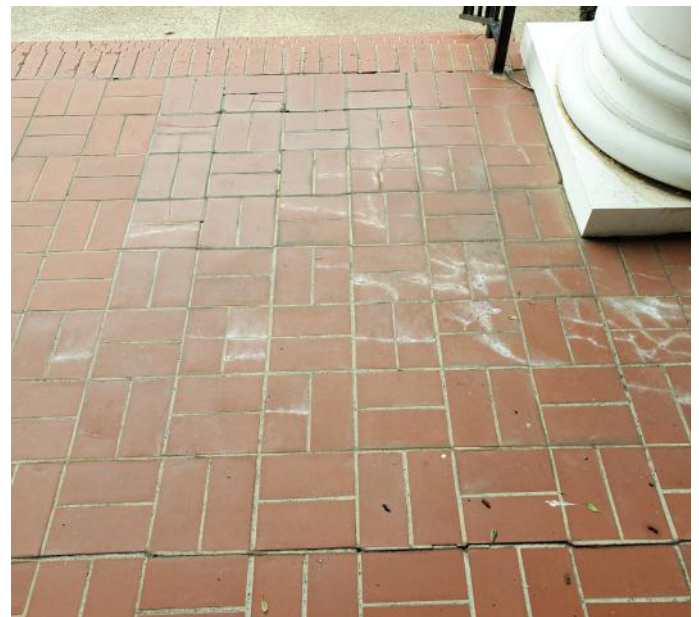
This exterior porch does not slope to the outside of the installation, causing water to pond, resulting in efflorescence. Note the cracked left-to-right grout joint, which should have been a movement joint with sealant.
