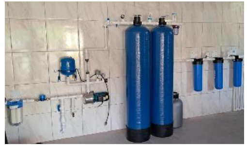
Water purification plant in San Esteban - Opened October 2024
