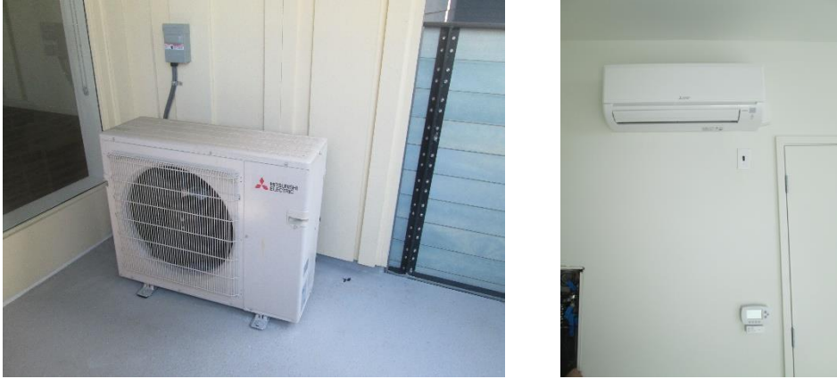
Figure 8. Ductless Minisplits Installed in Units
