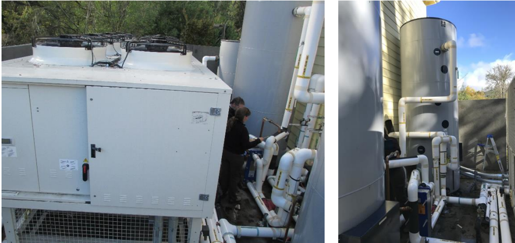
Figure 2. Aermec Installation at Calistoga
