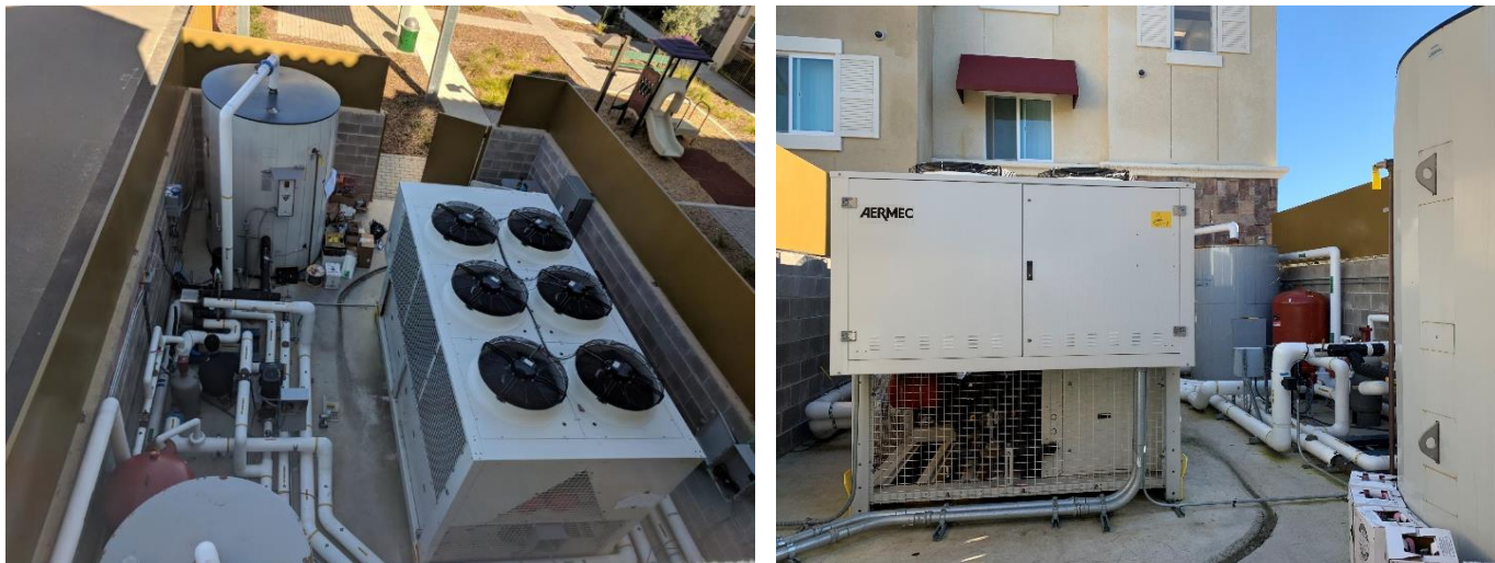
Figure 3. Aermec Installation at Cloverdale
