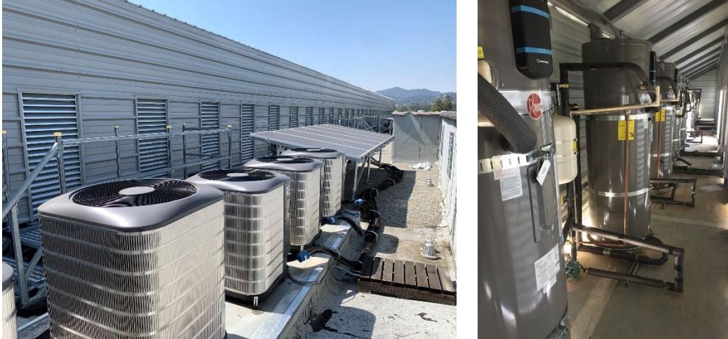
Figure 5. Rooftop Location for HVAC Outdoor Units and Heat Pump Water Heaters
