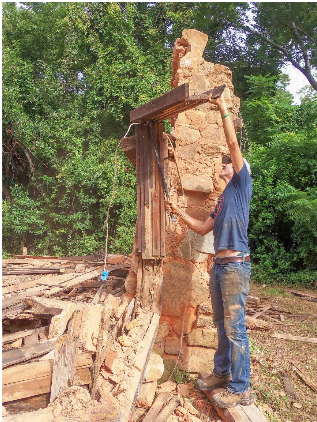
The Abbeville County Historical Society is in the process of working on the Creswell Cabin behind the Abbeville County Museum in Abbeville. Here is Steven Marnier hard at work this week on the cabin. The plan is to disassemble the cabin, which is in need of repairs, and assemble it again. It will be completely reconstructed, said Society president Andrew Hartsfield. Any rotten or split logs will be replaced. A donor here in Abbeville has volunteered to help fund the project. “We really would like to have the building put together by the early spring of next year,” said Hartsfield. (Staff photo by Henry E. Green)
