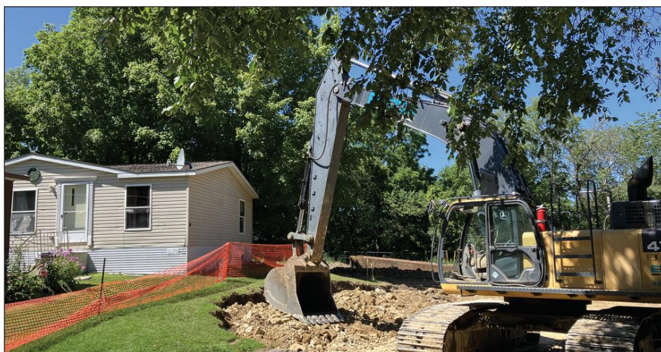
Zumbro Ridge installed several catch basins to redirect stormwater from their roads, one of several infrastructure improvement projects completed in recent years. Before the catch basins, the Co-op routinely spent thousands of dollars fixing road failure and erosion caused by stormwater.
