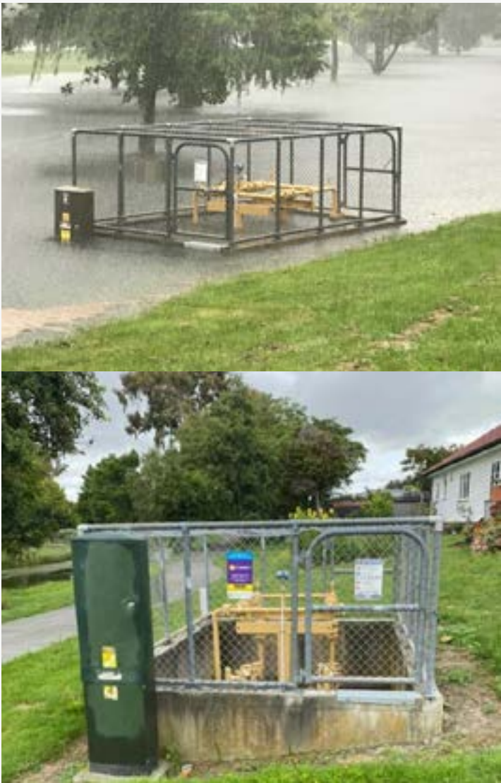
Images show a gas district regulator station in Hawke's Bay impacted by flooding. Mitigation of raising the communications cabinet has been carried out for improved flood resilience.
