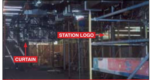
INSTALLATION AT KING'S CROSS UNDERGROUND STATION, LONDON, ENGLAND
