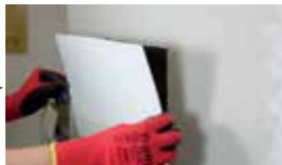
Adhere the paper to the plaster. Leave for 2 hours and apply 2 coats of EP/CP at 8m2 per litre per coat.
