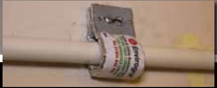
FCSS is suitable for protecting plastic conduit over doorways.
