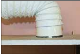
Flexible pipe can be pulled through the hole, rested onto the CLVM & pushed up into the ceiling
