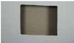
Clean off any loose parts of the plaster and measure the hole.
