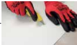
Cut the patch paper to the shape of the created hole, allowing 60mm round the outside for overlap.
