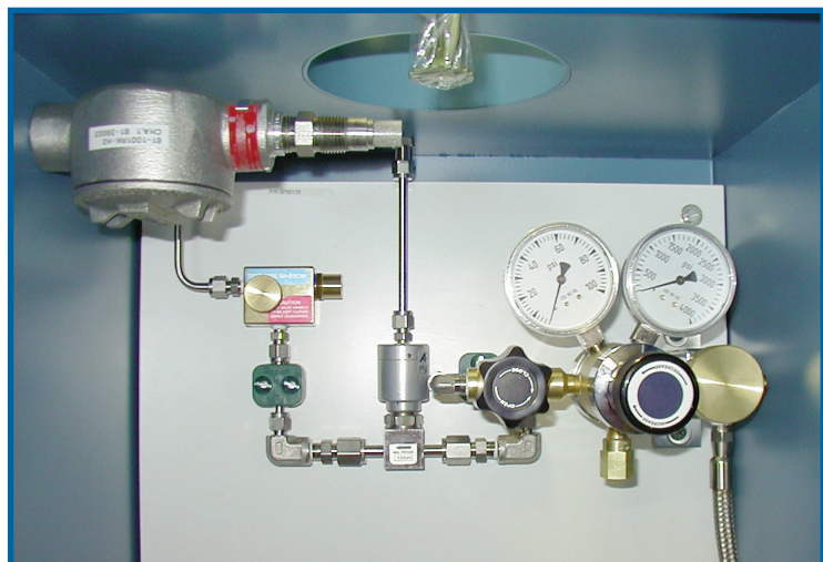
Hydrogen Gas Cabinet with Controls
