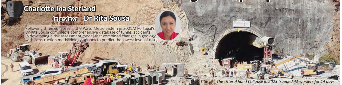
Title pic: The Utterakhand Collapse in 2023 trapped 41 workers for 14 days.
