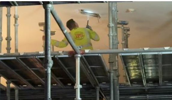
Another look at that light from below. They are getting ready for the next step of shoring.
