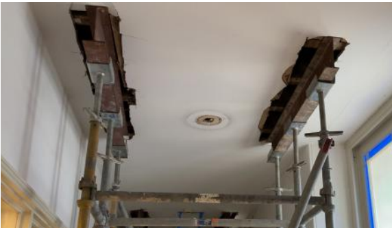
Notice how the steel I-beams are bracing the Sanctuary floor joists above.
