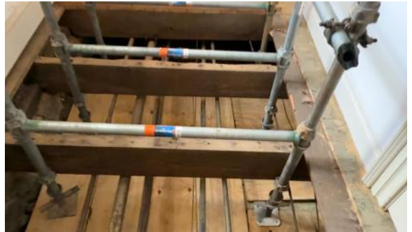
This is the view from the Chapel hallway after they built the foundation for the rigging to stand on.
