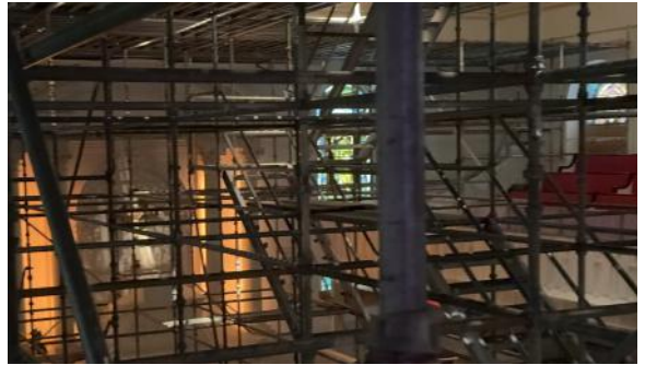
Further along with the installation - can you see the stairs in the middle?
