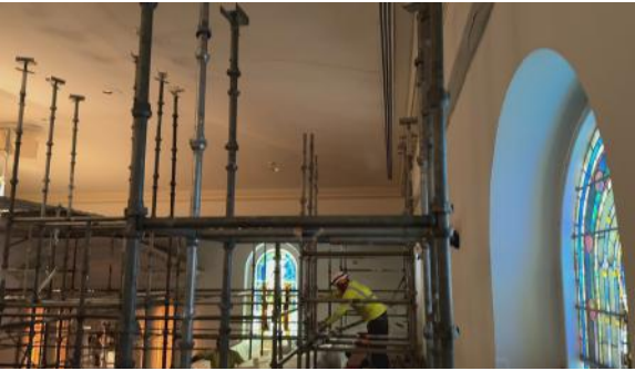
Here is a view from the balcony with most of the shoring in place.
