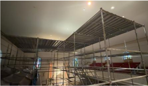
Once they reach the top level a floor is installed where they will work and is known as the “dance floor.”
