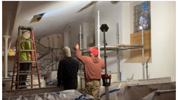
Shoring continued on the main level of the Sanctuary and will extend into the balcony.
