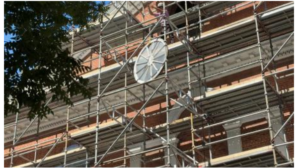
Outside the oculus window on the East wall was hoisted down to be restored.
