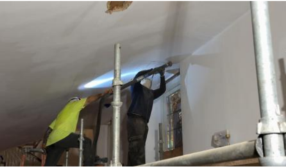
Cutting another section for the front rigging to be able to brace the balcony.
