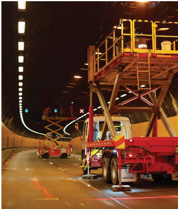
Terrace Tunnel maintenance work taking place. The tunnel will be closed at night from 8 to 12 February for its annual warrant of fitness check. Photo: Supplied.
