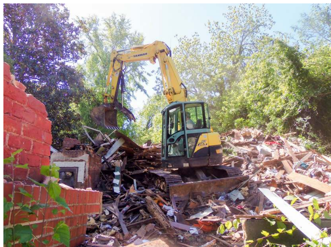
Houses in Abbeville can be condemned for a number of reasons. Here is one on Branch Street being demolished earlier this year. (Staff photo by Henry E. Green)
