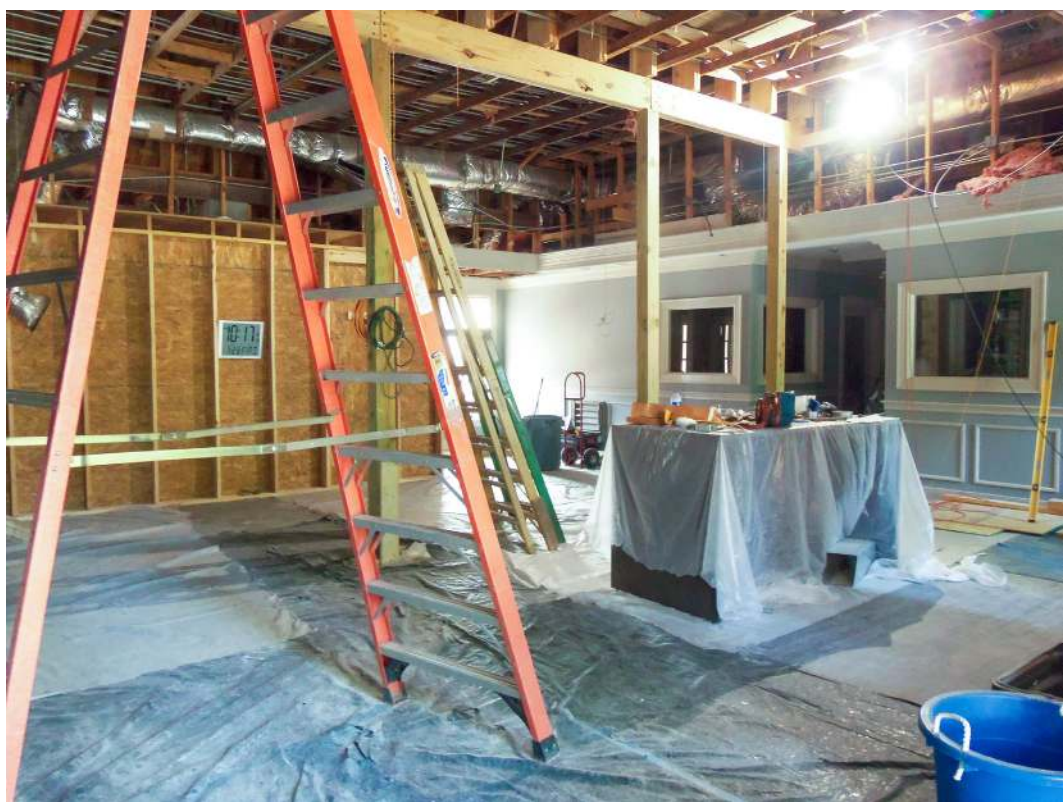
The lobby of Abbeville First Bank is currently closed, as is the drive-through, as the institution copes with the process of making major repairs in response to structural concerns. (Staff photo by Henry E. Green)
