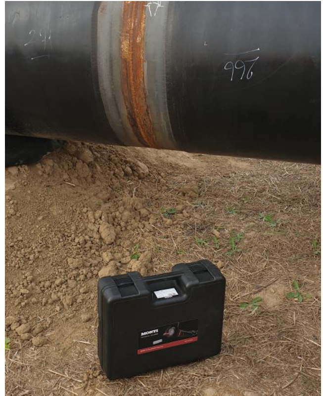
Figure 4. Training on the job before coating. MONTI's toolbox is ready for use.
