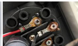
Malfunction due to corrosion
