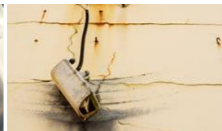
Loosen installation due to corrosion
