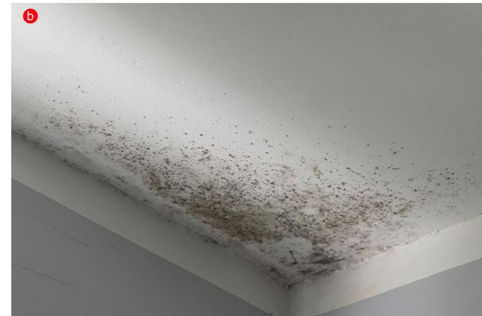
Black mould on living room ceiling under area of communal roof of 6th floor escape balcony
