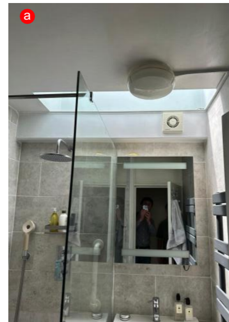
Rooflight over bathroom and extract fan (light switch activated)
