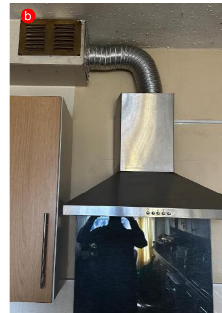
Kitchen extract potentially running into MVHR unit
