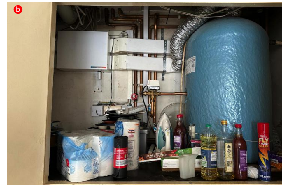
Kitchen utility cupboard with MVHR ventilation unit and ductwork, and hot water cylinder
