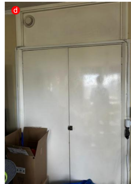
Living room supply air register over store
