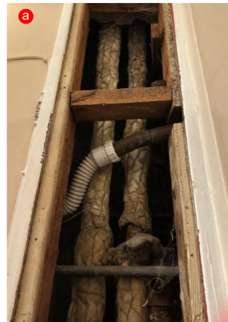
Service riser in entrance lobby with repair copper waste pipe
