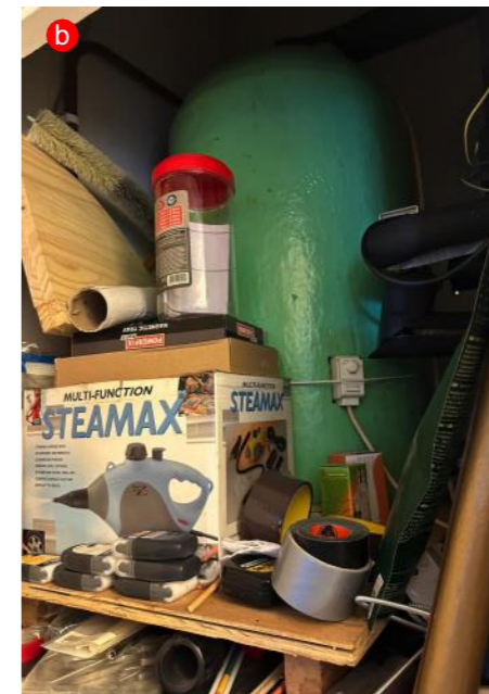
Hot water tank in hallway cupboard
