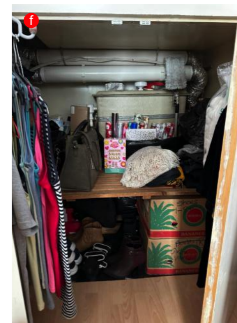
Bedroom utility cupboard with header tank and MVHR ductwork
