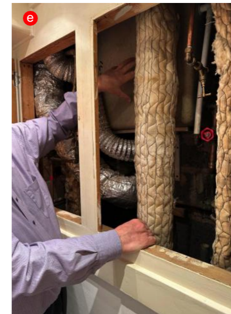
Service duct (WC) ventilation ductwork with unclear function and connection
