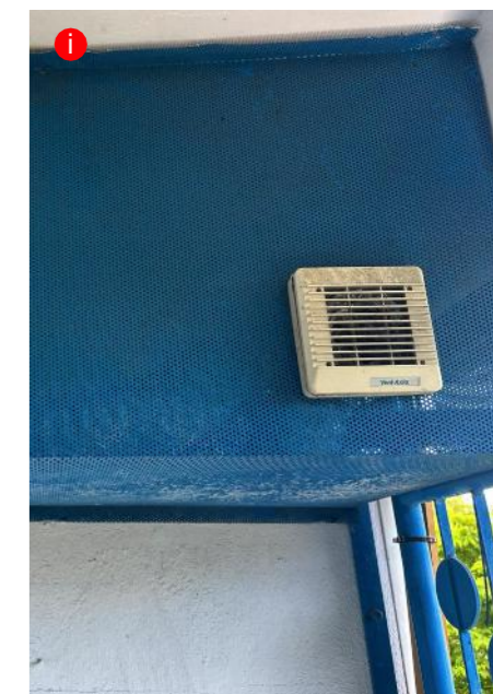
MVHR external air register in service cage at external terrace
