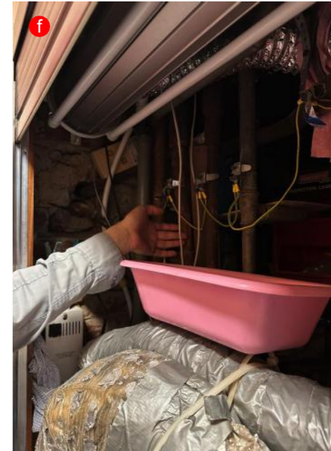
Historic district heating system pipework, now defunct
