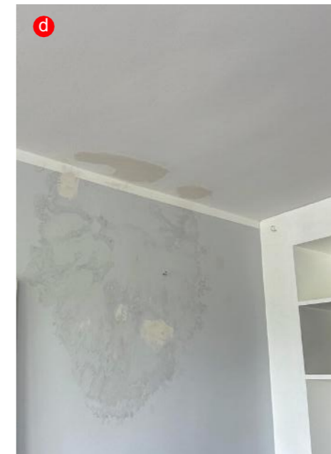
Water damage in living room under upper floor service duct
