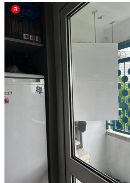
Gas combi boiler in external terrace
