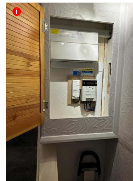
Electrical service head, meter and distribution board
