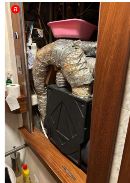
MVHR unit and ventilation ducts in WC service duct
