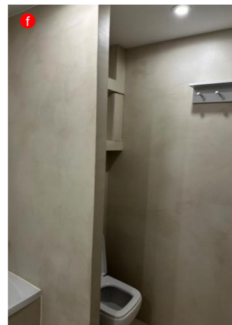
WC with no extract ventilation
