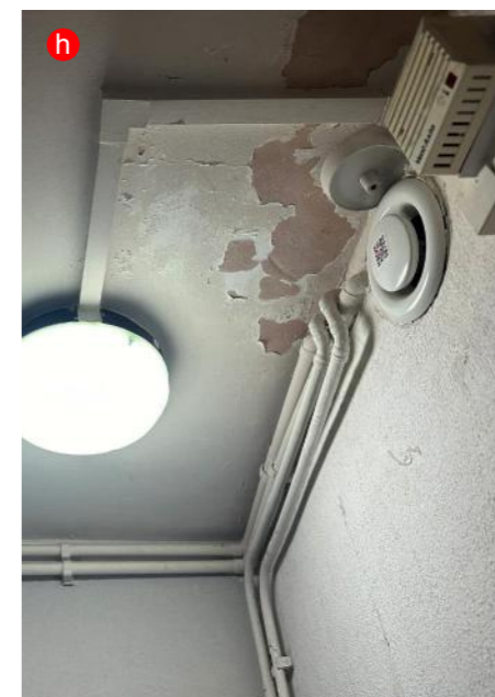
Non-operable extract register and condensation damage in WC
