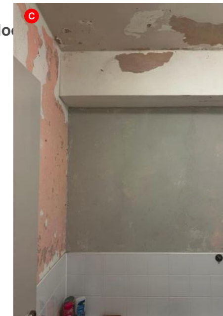
Extensive condensation damage to finishes in bathroom
