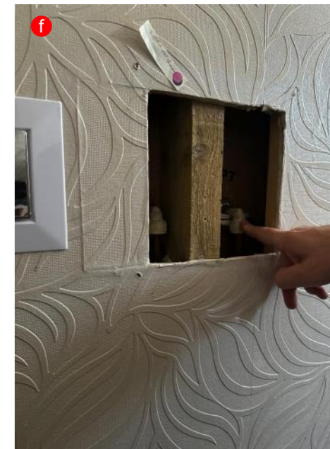
Power shower control panel in hallway
