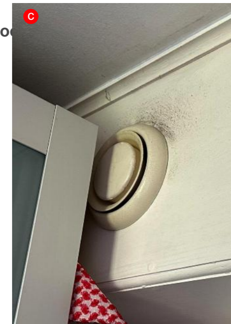
Supply air register with evidence of dirt/mould discharge
