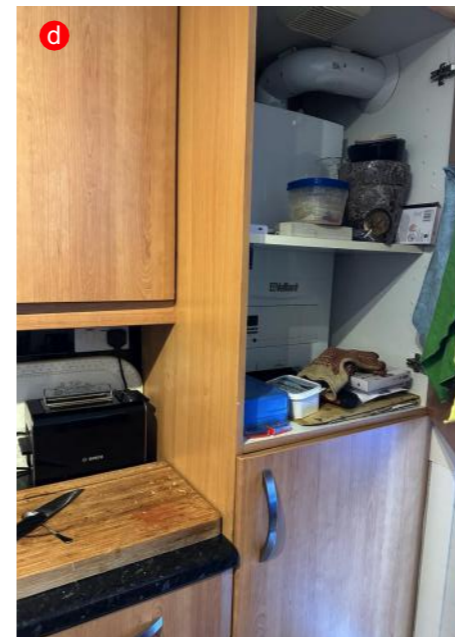
Gas boiler in kitchen with flue to external terrace
