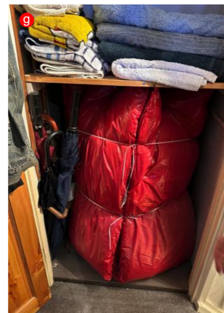
Hot water tank in hallway cupboard
