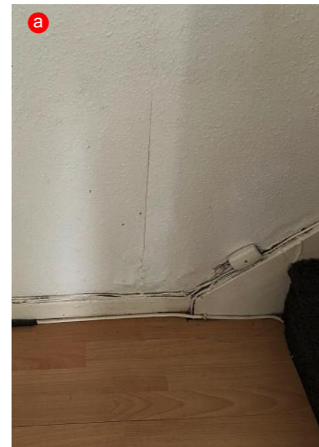
Damp ingress along partition with access corridor
