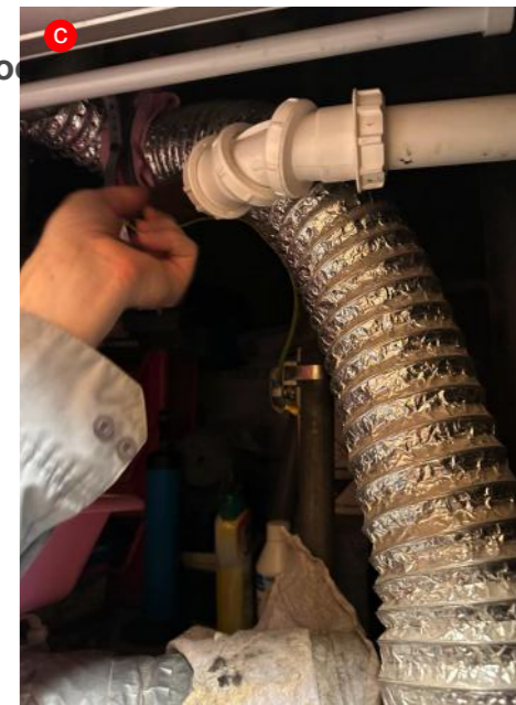
Failed copper pipework repaired with plastic in WC service duct
