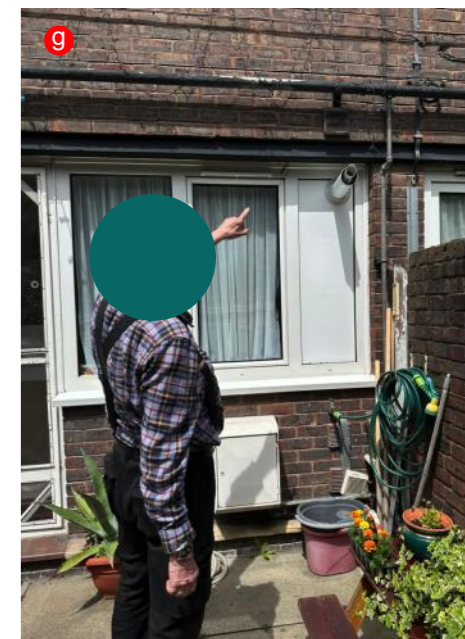
Garden elevation with boiler flue, MVHR intake/extract and gas meter
