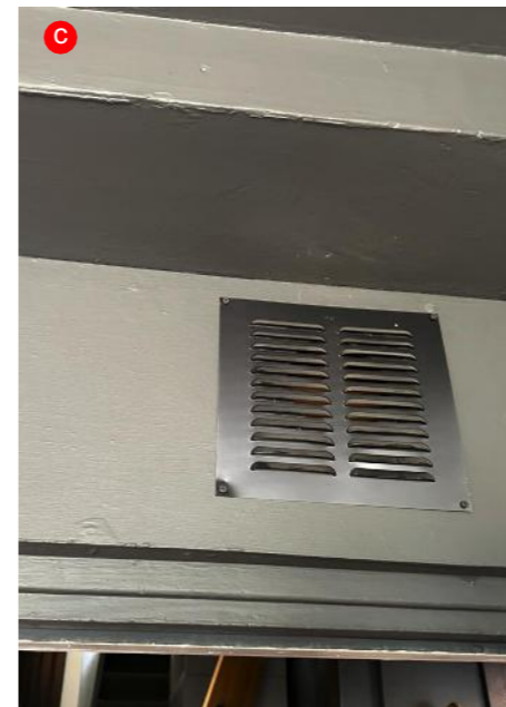
Ventilation grille, defunct (no mechanical ventilation in property)
