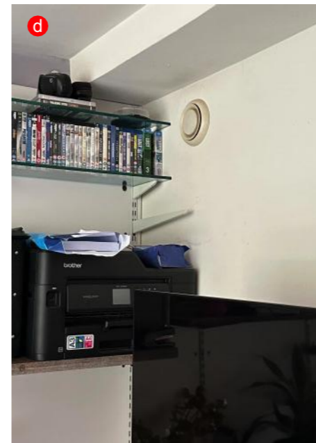
Active supply air register in living room
