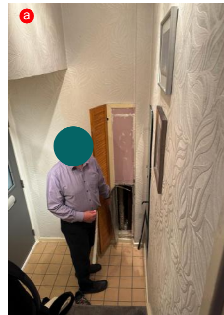
Service riser and access panel in entrance lobby
