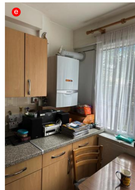
Gas boiler in kitchen with flue to garden
