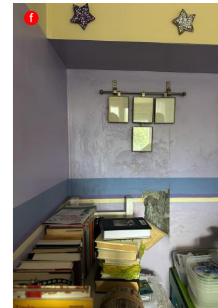
Damp/condensation damage in master bedroom at separating wall
