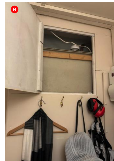
Header tank in hallway cupboard
