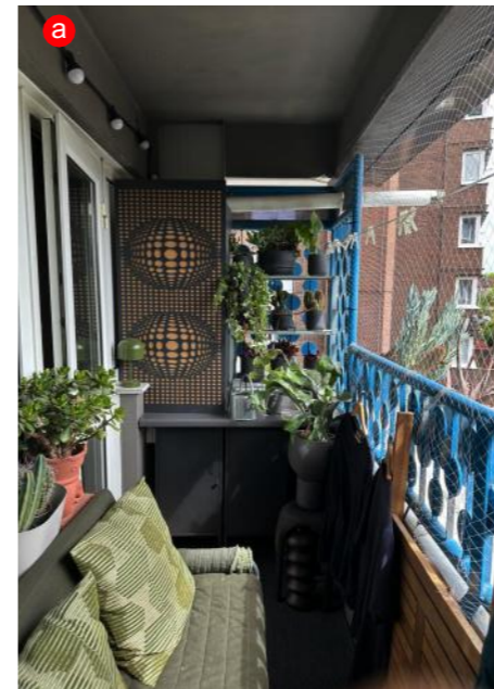
External cabinet on terrace housing gas Combi boiler
