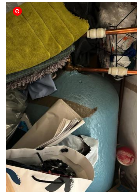
Hot water tank in hallway cupboard
