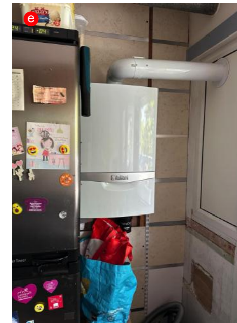
Gas combi boiler with flue to external terrace
