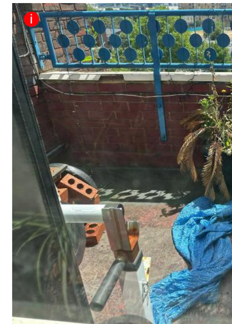
Kitchen terrace with poor drainage issues
