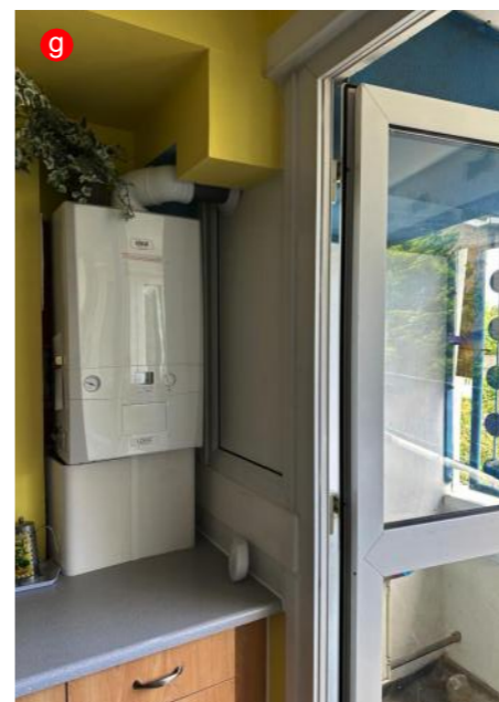
Gas boiler with flue to external terrace
