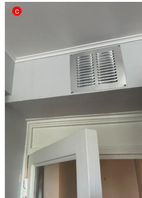
Defunct ventilation grille, ventilation installation has been stripped out
