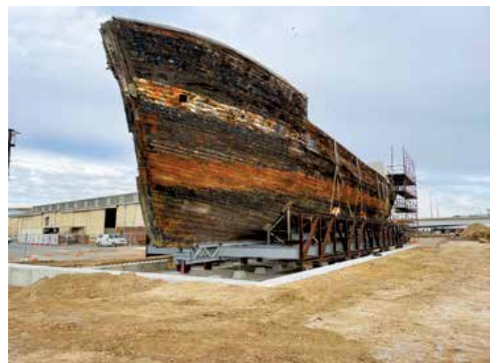
The ship in its final position, still to be lowered onto foundations
