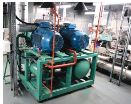
The 707kW BITZER Ammonia Compressor Pack (ACP), powered by high performance screw compressors, at Pilgrim UK's Bromborough site
