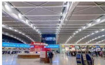
LED airport lighting (Source: ENELTEC)
