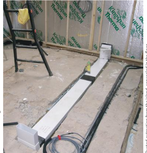
Ducted extraction from the island, concealed in the floor.
