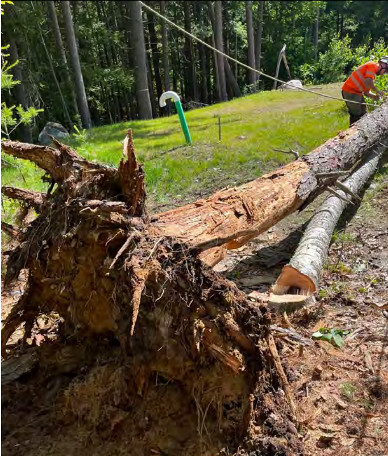
Photo 13: Hemlock stump uprooted during the lowering procedure, leaving hinge and back cut intact and showing just how compromised the tree had been, prior to removal.
