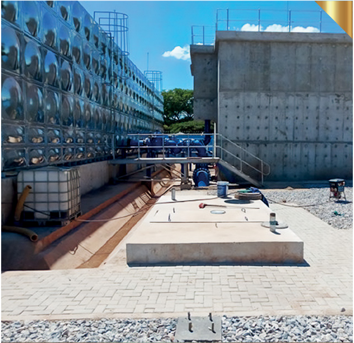
Chelston DC Steel tank & Contact Tank
