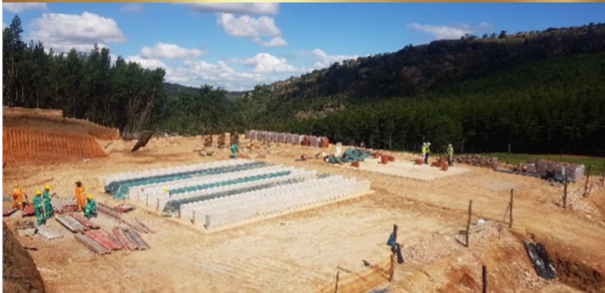
Reservoir base & Structural Steel placement and fixing on the Eswatini Water Supply Access Project
