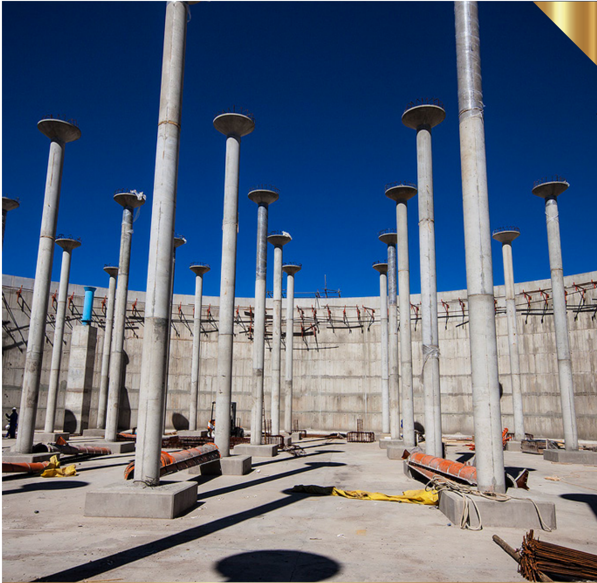
Jane Furse Reservoir: The completed reinforced concrete (RC) circular wall and columns with conical column heads are ready to support the cast-in-situ RC roof slab.
