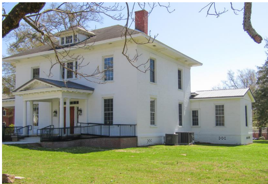
Erskine's Alumni House, located in downtown Due West, has been getting a very serious makeover. (Staff photo by Henry E. Green)
