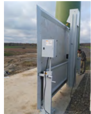
Box for protecting the control
