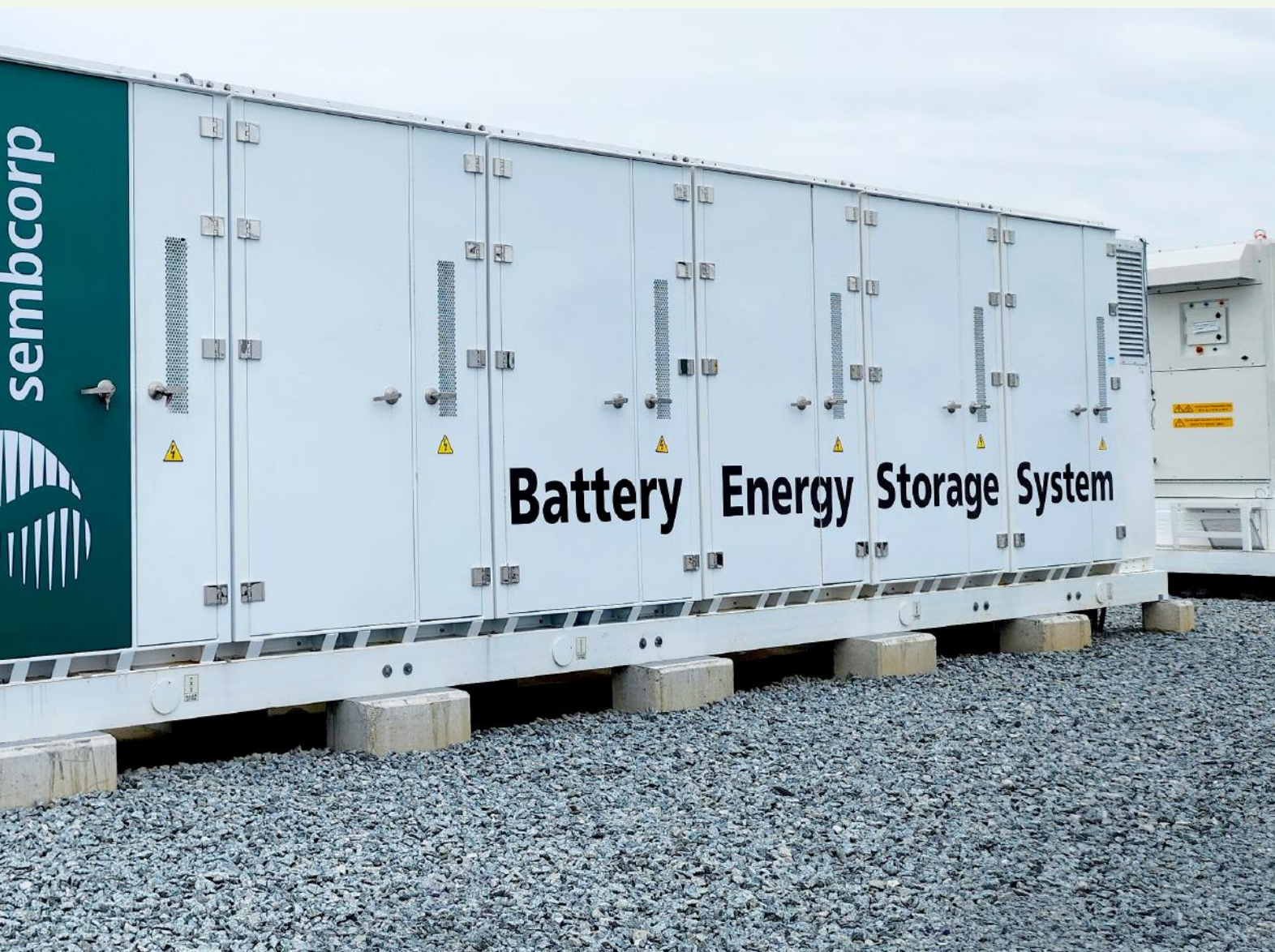
The 285MWh Sembcorp Energy Storage System spans across two hectares of land in the Banyan and Sakra region on Jurong Island.
