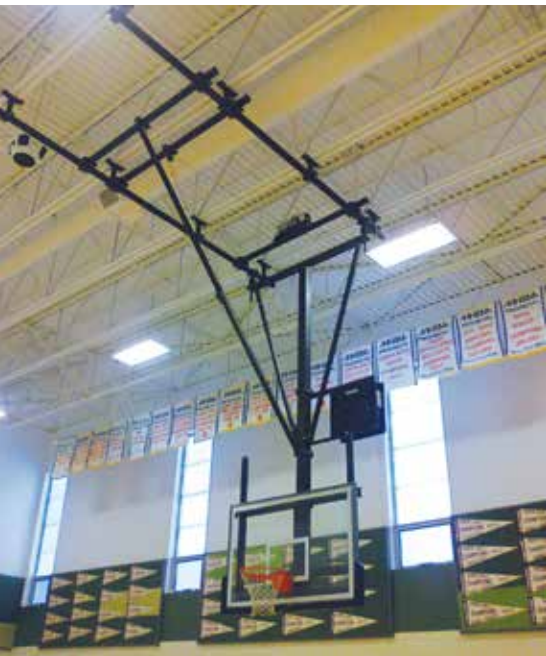
Indoor equipment inspections which entail preventive maintenance can ensure the longevity of equipment, eliminate costly emergency repairs and keep users and personnel out of harm's way.
