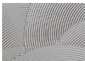
NO Incorrect application
