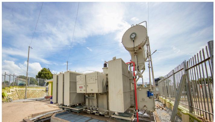
Nakasamba substation, Entebbe
