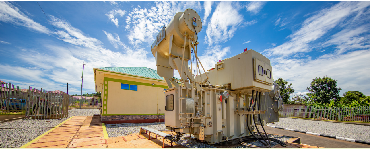
Kakiri Substation, Wakiso District.
