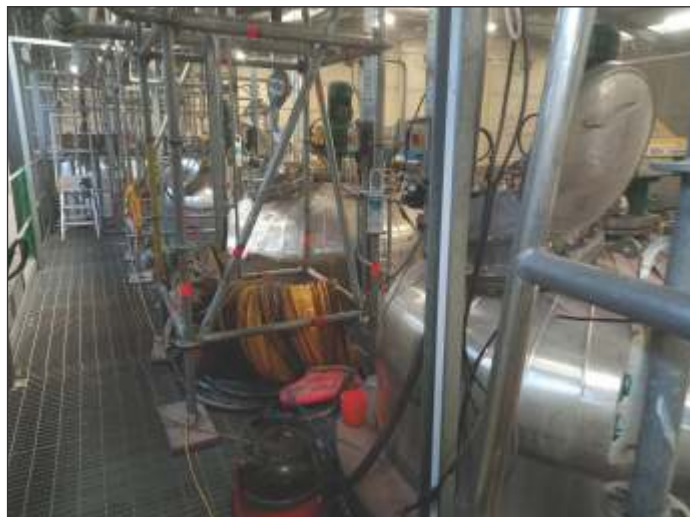
Figure 1: High-performance coating required to protect tanks against corrosion.
