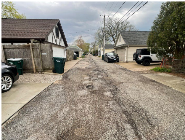
Alley #3-38 (Serious) Located between Highland Ave and Washington Ave Entrances at 16 th St and 15 th St
