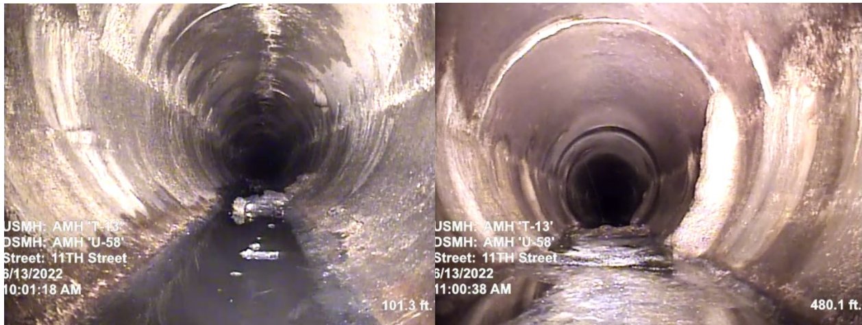
Fractures and Deposits in the Central-Greenleaf Alley Sewer
