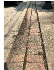
Brick settlement behind curb
