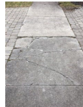
Cracking with Displacement
