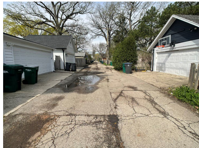
Alley #2-37 (Very Poor) Located between Maple Ave and Laurel Ave Entrances at Crescent Pl and 6 th St
