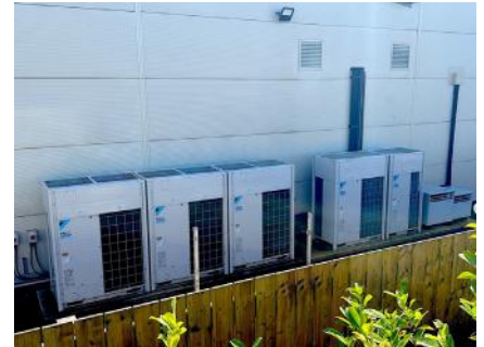
Daikin heat pump-based VRV outdoor units alongside the centre
