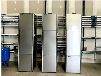
Plant room with hot water systems and associated pipework
