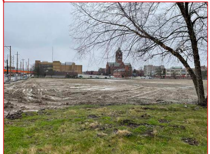
View of the Former Hospital Site after demolition from Chicago St. facing northeast between Lincolnway and State St.
