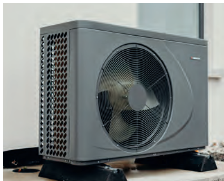
Efficient heating for a new build bungalow in Glenavy
