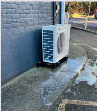
The hazards when your install does not have adequate condensate removal
