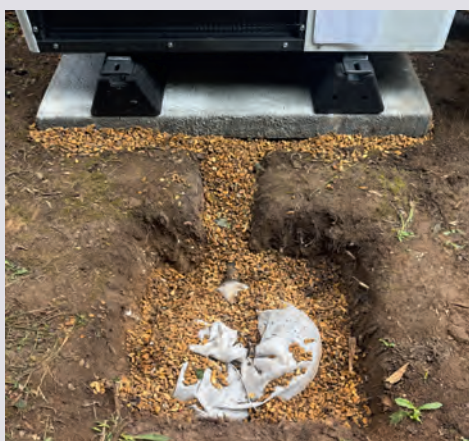
The DiversiTech ASHP Soak-Away in the ground ready for the completion of the installation
