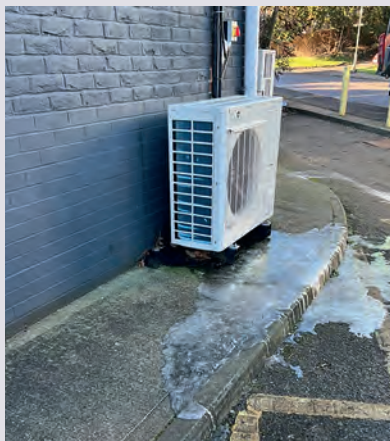
The hazards when your install does not have adequate condensate removal
