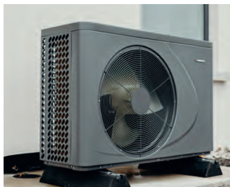
Efficient heating for a new build bungalow in Glenavy P24
