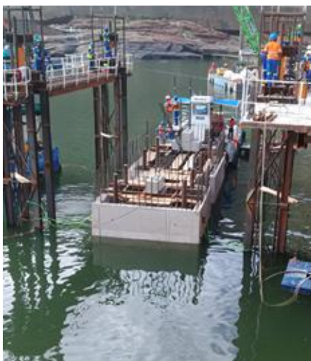
The piers were slip-formed as hollow structures, from a specially-built rig in the Zambezi River. Photo credit: Peri Formwork and Scaffolding
