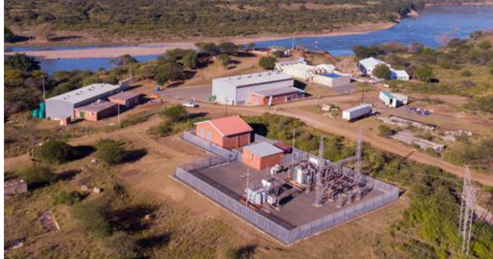
The pump station abstracts raw water directly from the Thukela River
