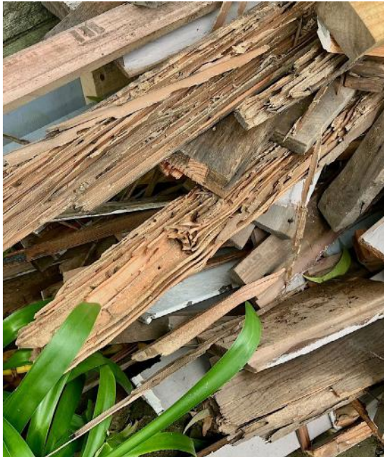
Photo: Termite damaged to be discarded
