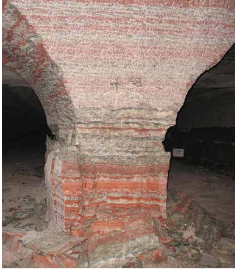
Typical pillar deterioration in a potash mine.
