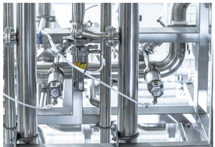
The steam trap at the leakage outlet is integrated into a closed drain piping system – efficient and hygienic. (photos: Evoguard)
