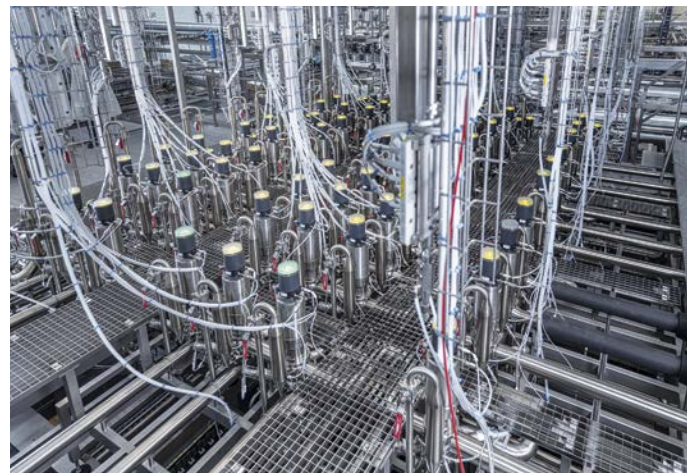
The new sterile manifold connects the tank farm with the filling lines – space-saving installation on an elevated platform
