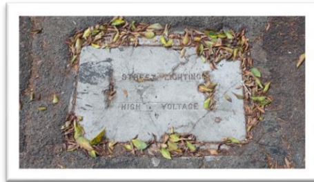
Concrete #VPCMc3 High Voltage
