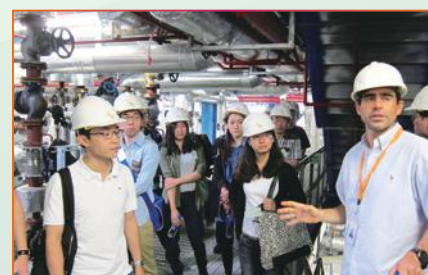
ASB Biodiesel Plant
