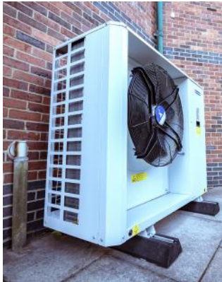
Tyneham heat pump system
