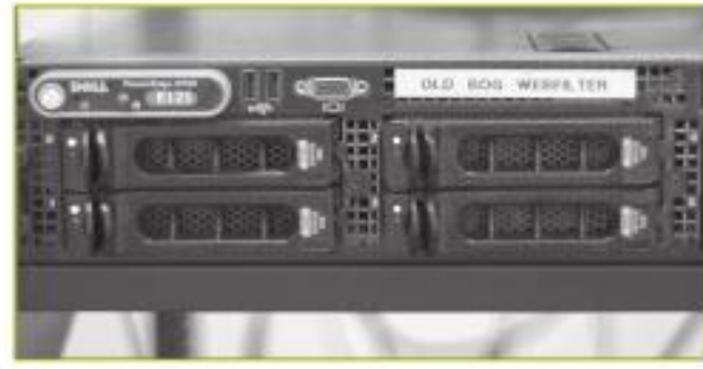
a section of our new rack, relocated to a safer place
