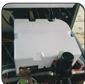
Power protection cover for safety
