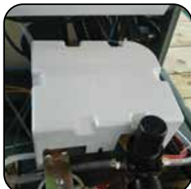
Power protection cover for safety
