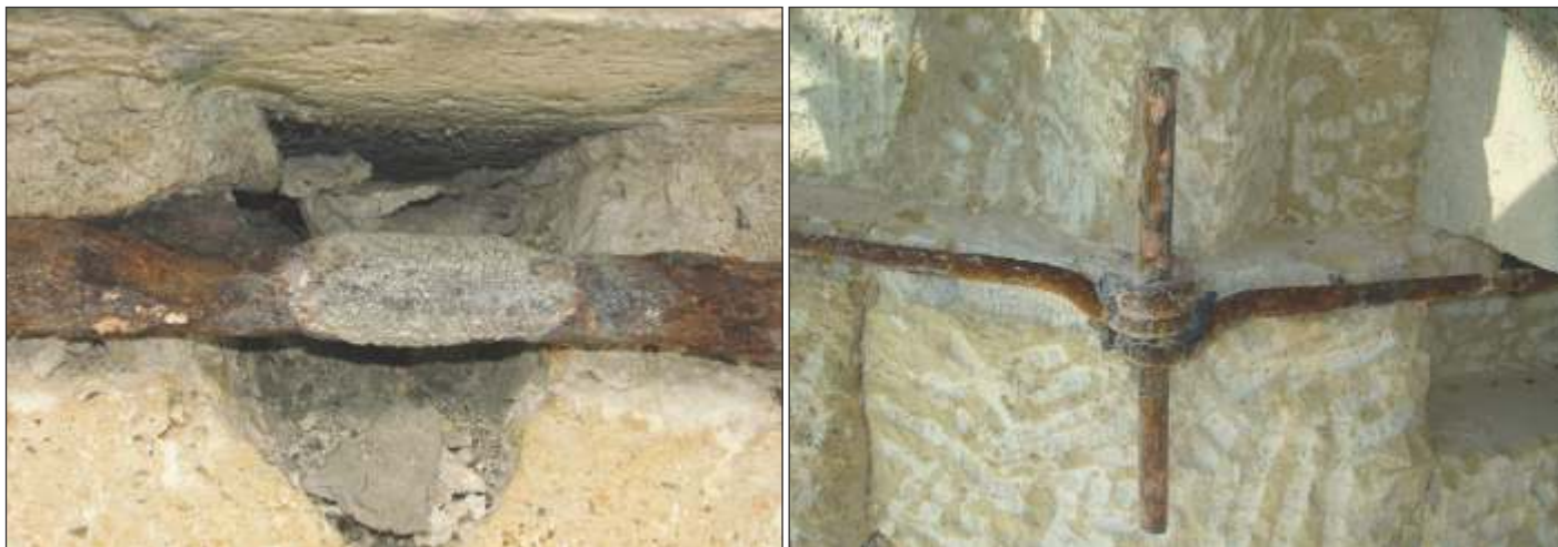
The joints were reinforced with steel fishplates that were welded onto the joints and also protected with CorrVerter® MCI® Rust Primer.
