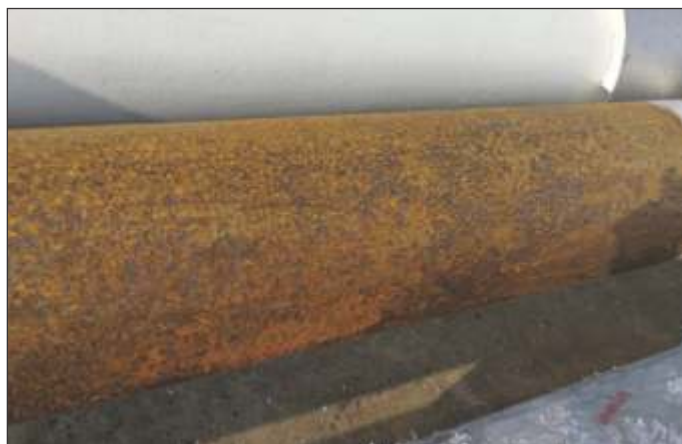
Image 2: Damaged pipeline after suffering from Corrosion Under Insulation (CUI).
