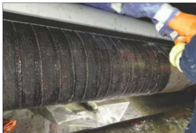
Image 3: After rebuilding the pipe to original profile using Belzona 1111, several wraps of Belzona 9381 were applied.
