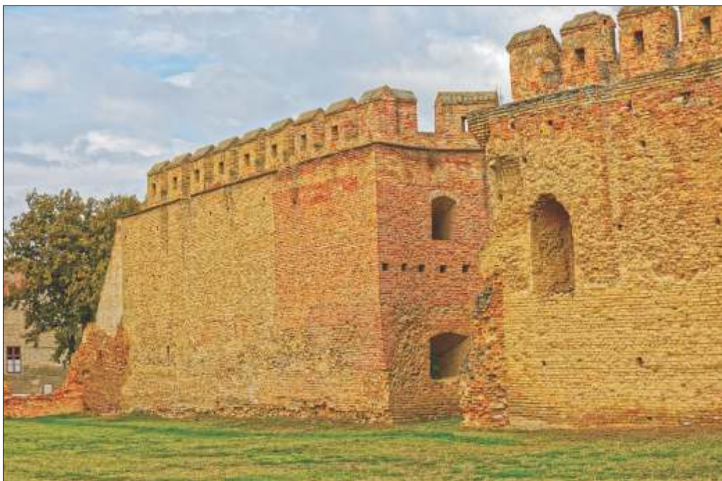
Renovation work includes strengthening of the foundations, restoration of collapsed parts, and injection of cracks.
