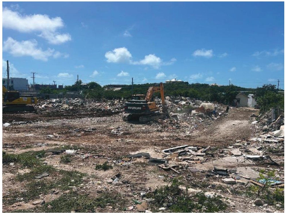
The cleared area of once used to be a densely populated unplanned community in the vicinity of the Caicos Lodge area of Providenciales
