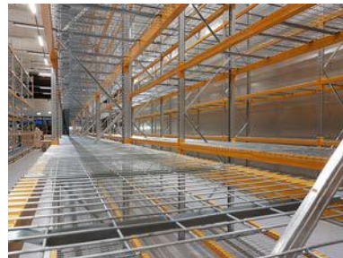
5 SHELVES Our sturdy shelves are made from steel mesh, which allows light as well as water from sprinklers to penetrate.
