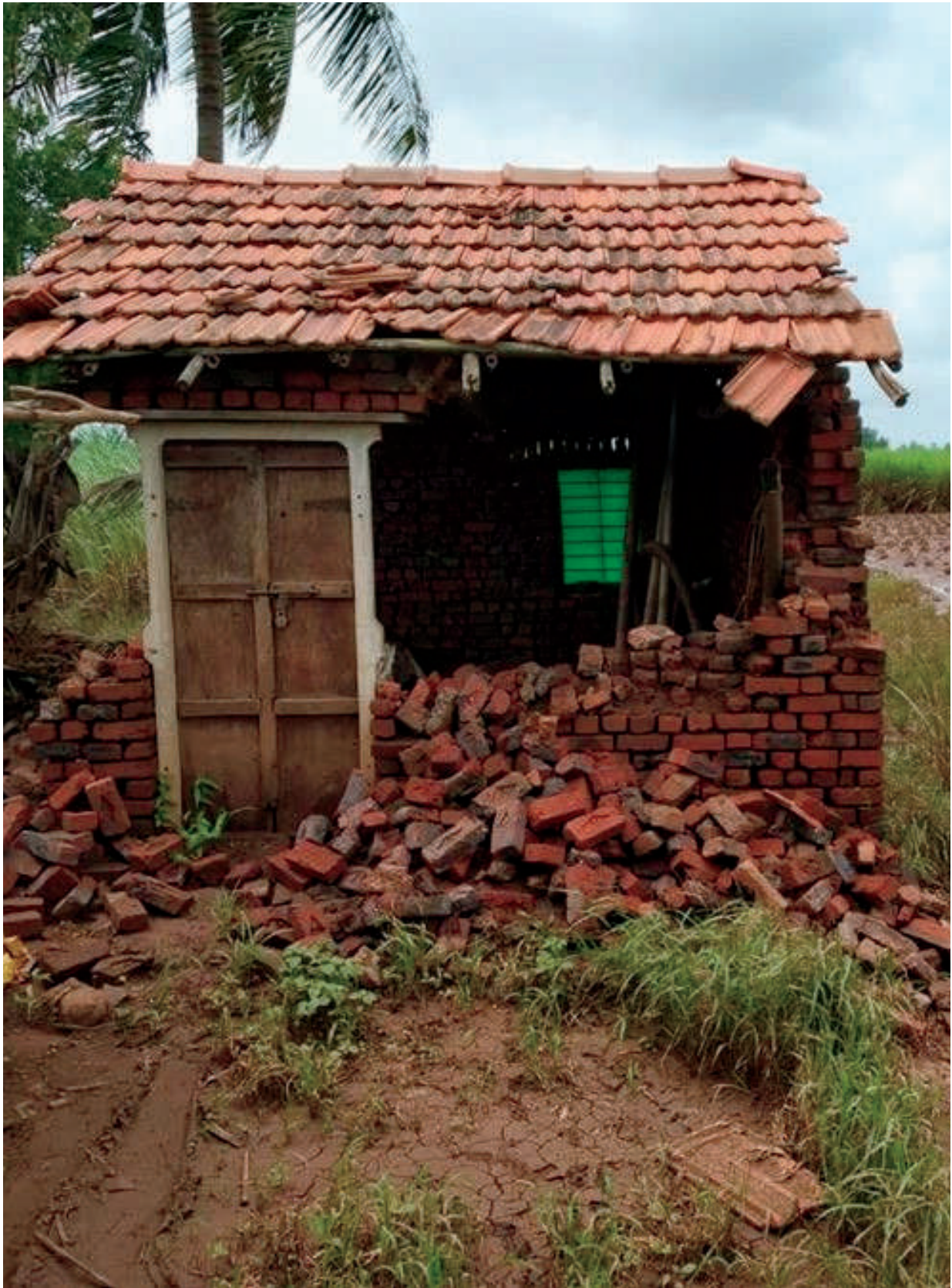
2019 flooding in Karnataka. Houses ruined by floodwaters
