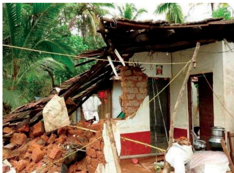
House damage situation after flood.
