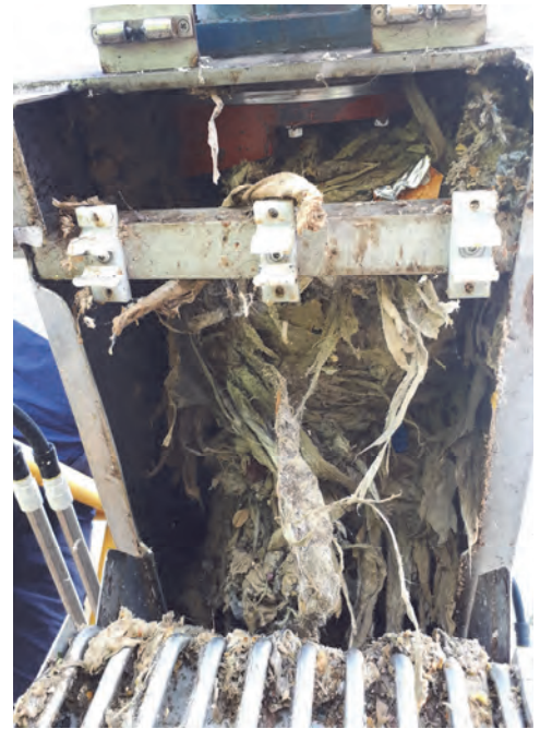
Below: Wet Wipes clogging up machinery
